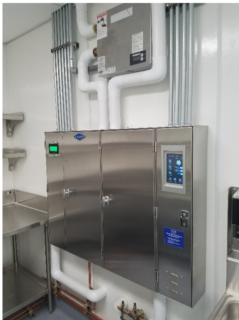
Figure 1-2-3 GPC-7000-SPC, Spray Odor Cabinet, and AirVantage Command Center
