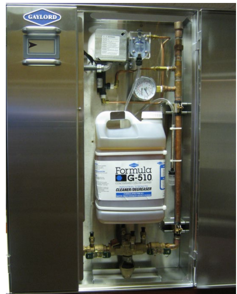
Figure 2-3-1 Wash Control Cabinet
